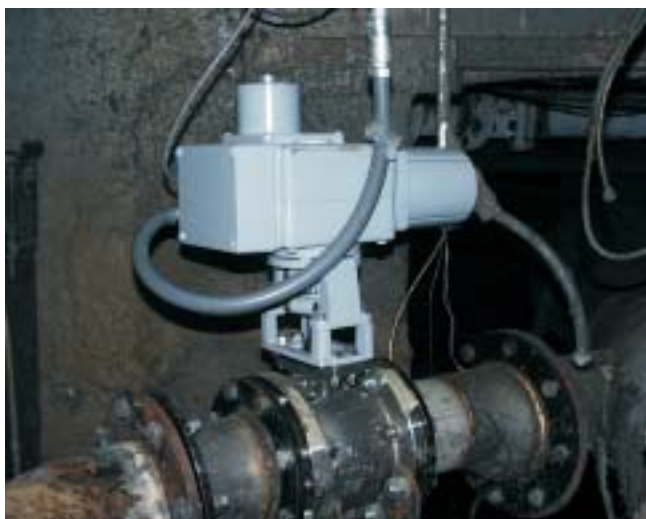
Vat level control valve
