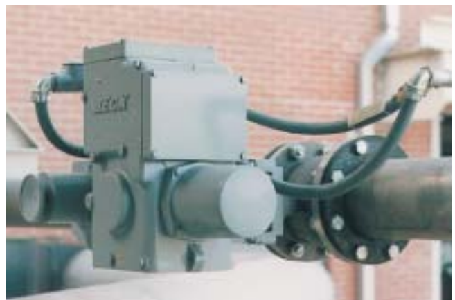
Refiner pressure control valve
