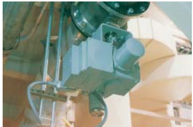
Stuffbox level control valve
