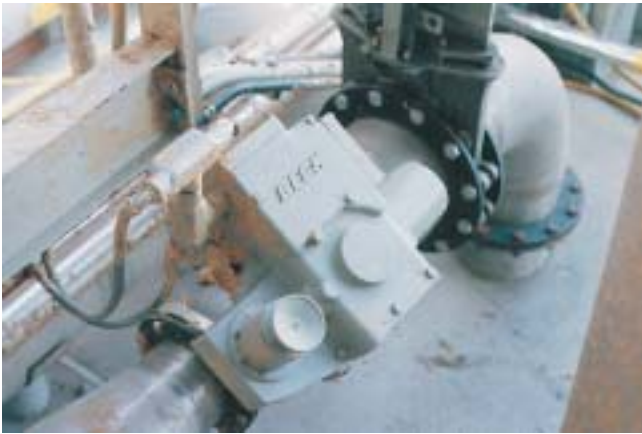
Machine chest recirculation control valve
