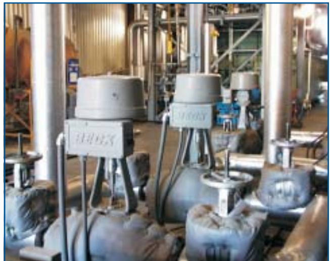
Group 14 linear drives on condensate return valves.
