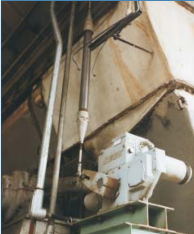
Beck replacement installed on an outdoor modulating FD fan damper. Note obsolete pneumatic lines.
