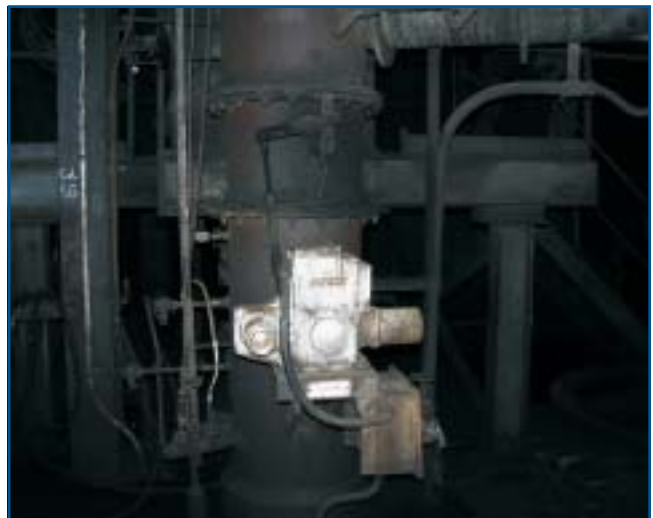
Beck drive installed on a coal mill exhaust damper.
