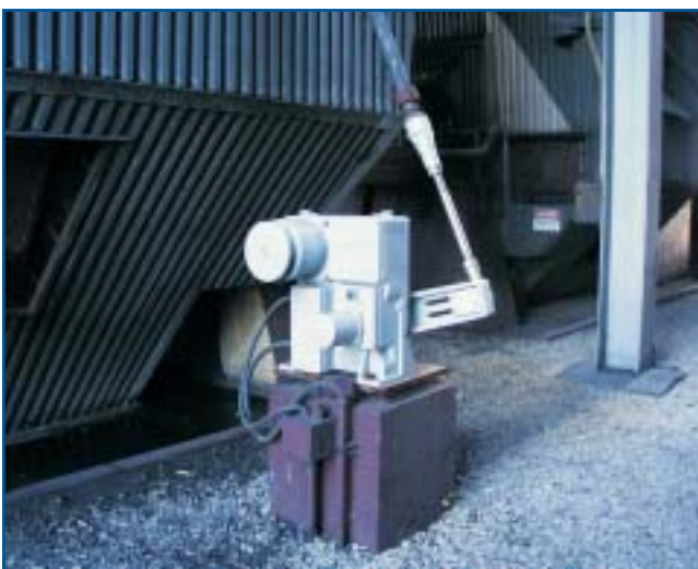
Beck Group 22 drive installed on a damper.
