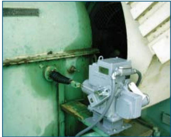
Raw Mill Dust Collector Fan Speed Control
