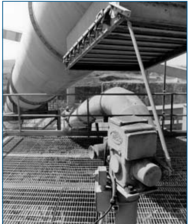
Baghouse Tempering Air Damper
