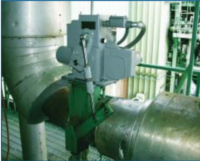
Main Fuel Gas Valve
