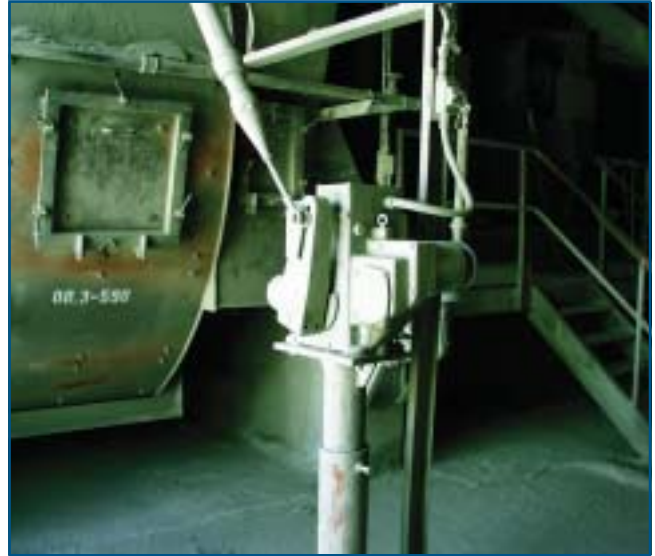
Primary Air Fan Damper
