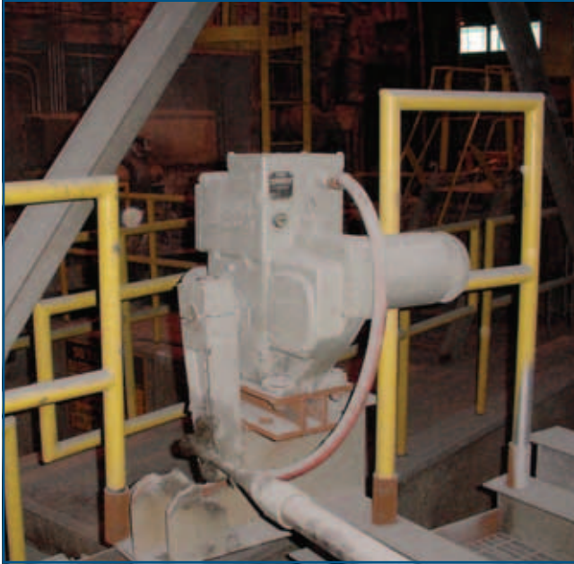
Furnace Combustion Air Damper
