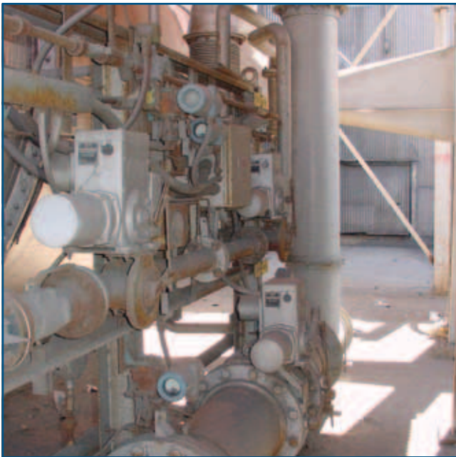
Pre-melt Furnace Gas & Air Valves
