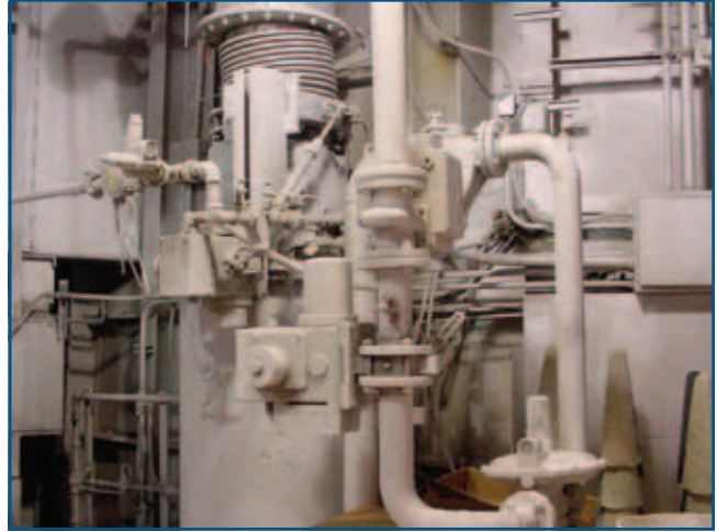
Melting Furnace Gas Valve
