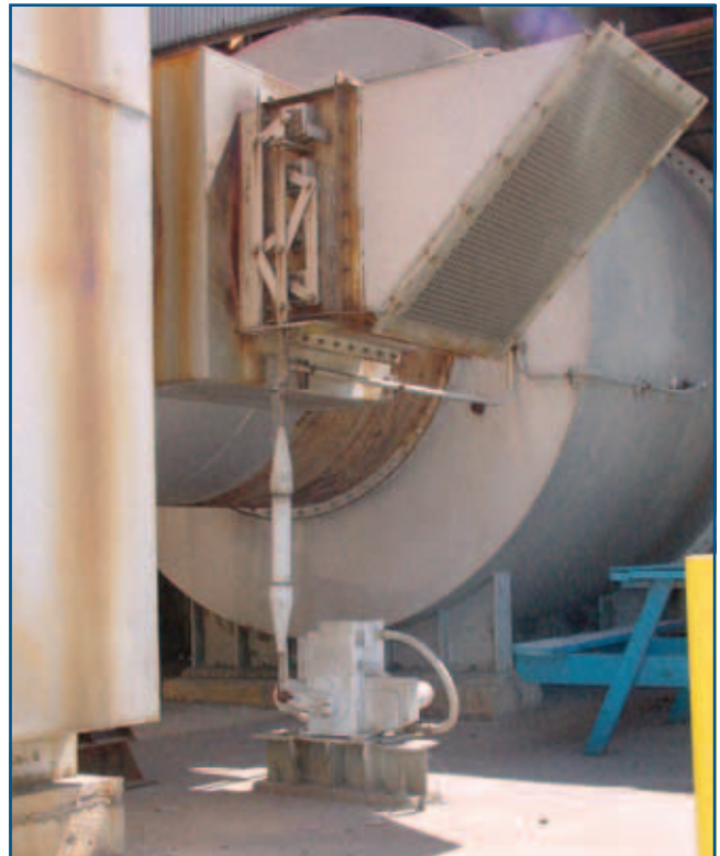
Mixing Air Bottom Damper
