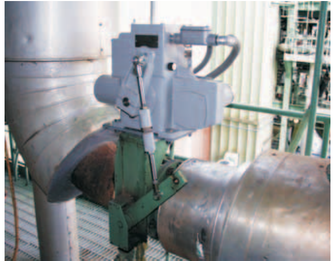
Group 11 drive on a main gas control valve (with linkage)
