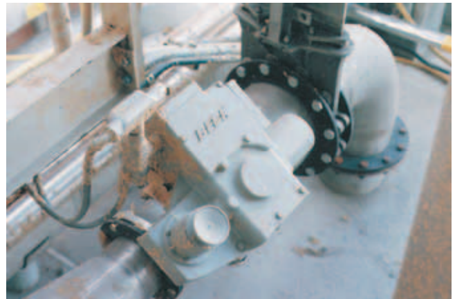
Machine chest recirculation control valve
