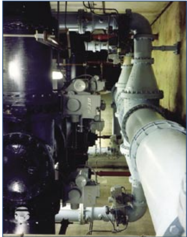
Multiple Beck drives on flow control valves
