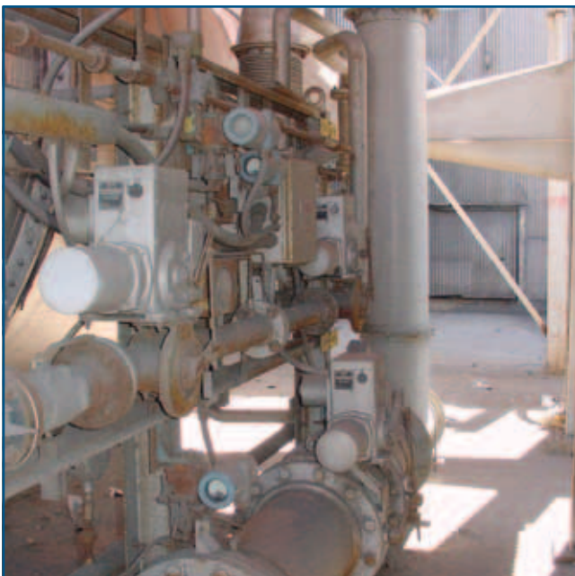
Pre-melt Furnace Gas & Air Valves
