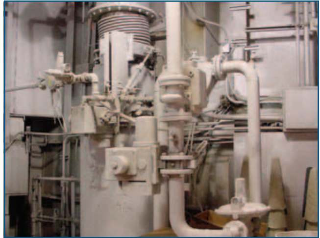
Melting Furnace Gas Valve
