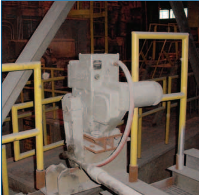
Furnace Combustion Air Damper
