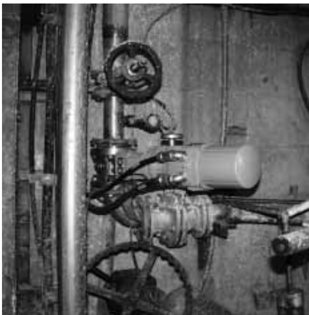
Model 31-M50 installed on a machine chest dilution control valve
